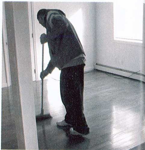
Photo courtesy of Major Homes | To help out a married couple with health issues, Major Homes remodeled a room, free of charge.
